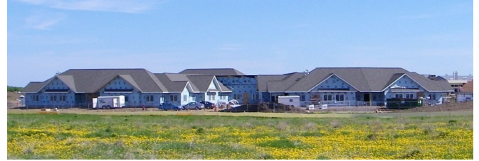
Christian Community Homes was awarded a $400,000 RBF Revolving Loan Fund loan. The funds assisted the development of this assisted living facility in Osceola, WI, helped leverage $8.5 million in private funds, and supported the creation of 49 jobs.
